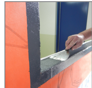
14. Allow VaproLiqui-Flash to set up until dry to the touch, then inspect for voids and apply additional VaproLiqui-Flash as needed to achieve complete coverage.
