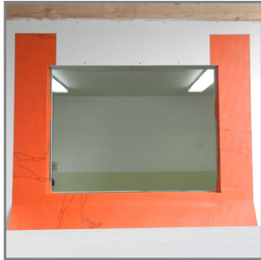
8. Install head flashing only after both left & right jamb pieces are fully adhered.
