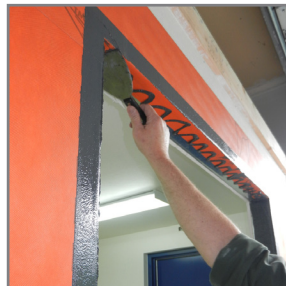
13. Immediately spread until all surfaces are completely covered and substrate below is no longer visible (approximately 12 to 15 wet mils).
